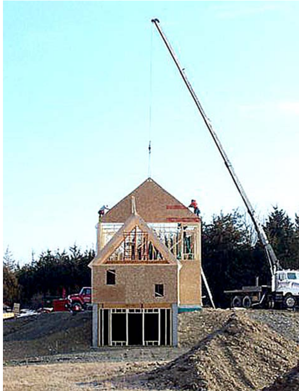
Hoisting the peak. There was a time, still observed in Europe, of crowning a new house with a small evergreen when the peak was first framed. Today, with mechanicals and assemblages galore, construction is a just-in-time assembly line requiring attentive management, too busy for ceremony.
